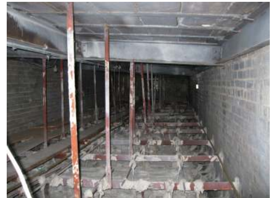
Mechanical Duct space in the attic of the Capitol
